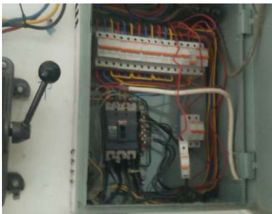
Gambar 5. Main Panel terbuka
