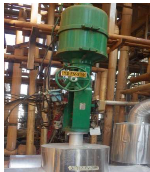
Gambar 4. Control valve 12 – FV – 219
