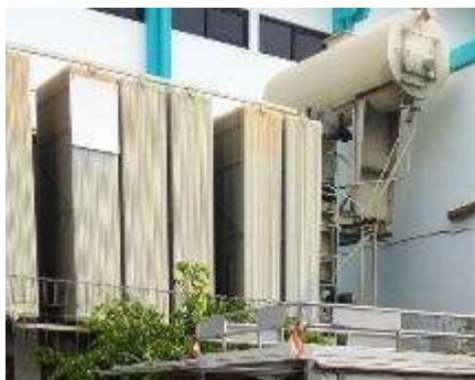
Gambar 6. PAUWELS power transformer 150kV/20kV
